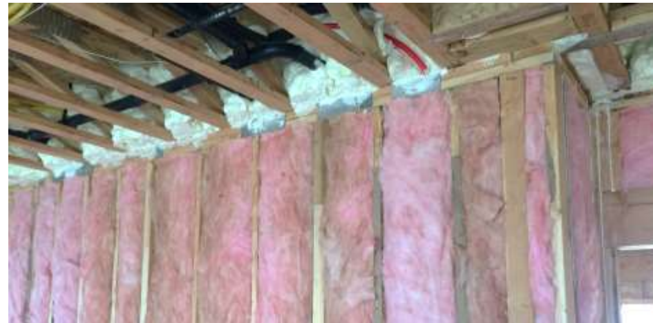
Foam at rim joist
